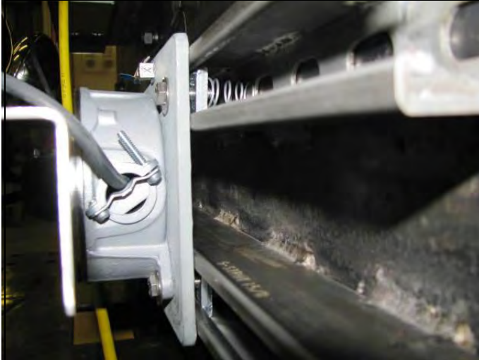
Mounting bolts (Qty 4) torqued to 78.5 in/lbs. on the 4634 units.
